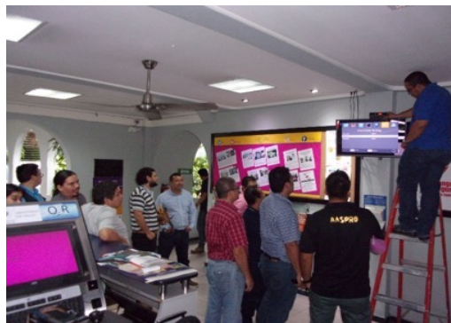
EWBS receiver installation at a government agency
