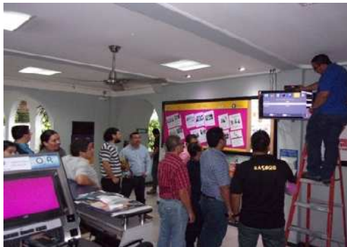
EWBS receiver installation at a government agency
